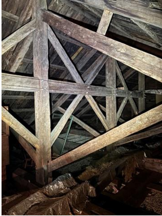
Photo 15: Missing brace in Main Truss
