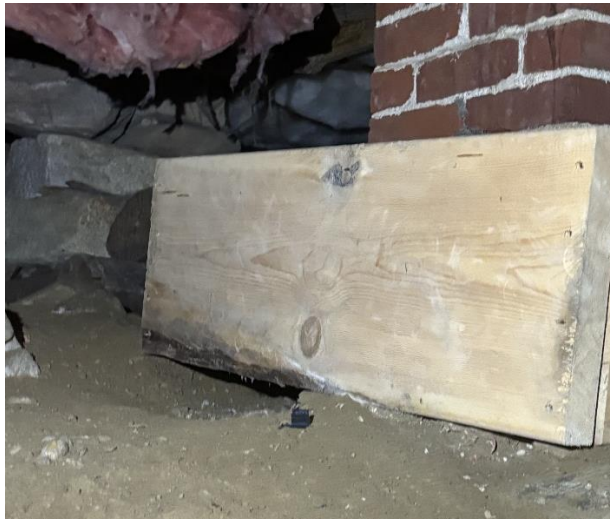
Photo 9: Burrow below pier
