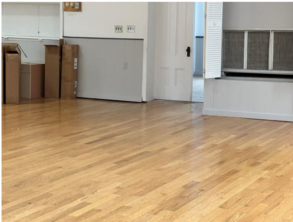
Photo 6: Deflection in Main Room Floor
