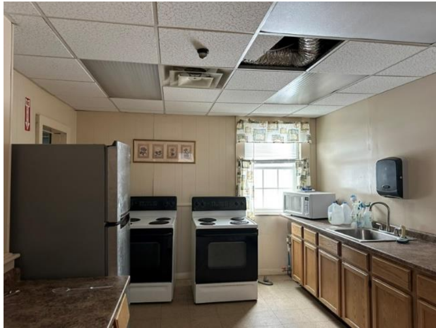
Photo 11: Deflection in Kitchen Ceiling
