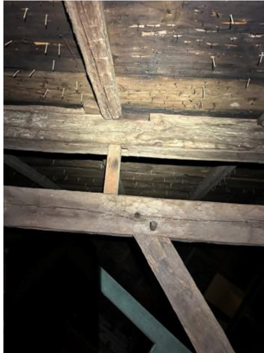
Photo 13: Multiple open notches throughout Main Truss chords
