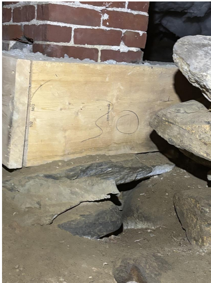
Photo 8: Burrow below pier
