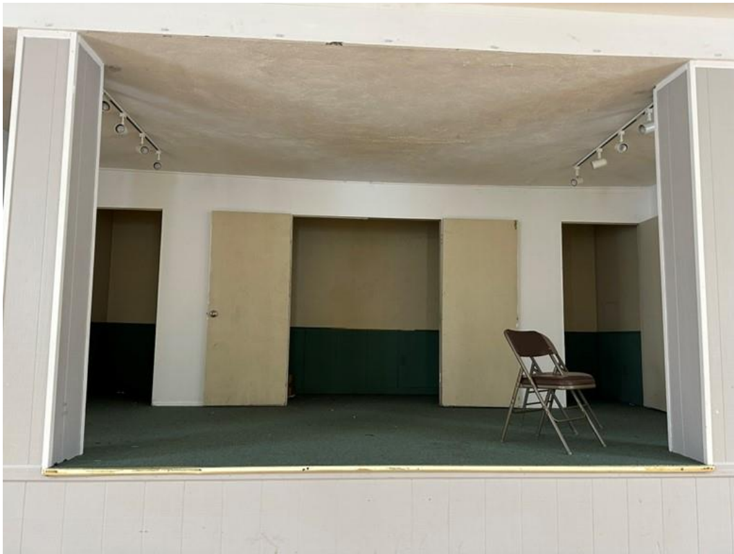
Photo 4: Deflection in Stage Ceiling
