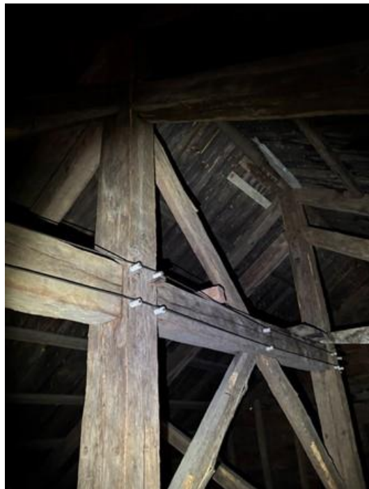
Photo 16: Missing brace in Main Truss
