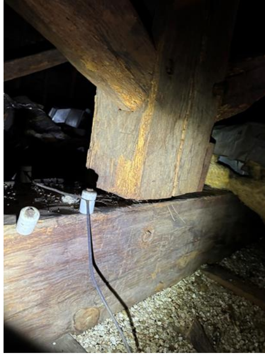
Photo 17: Powderpost beetle damage to trusswork
