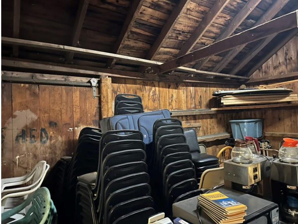
Photo 3: Deflection in Wall Plate of Side Room
