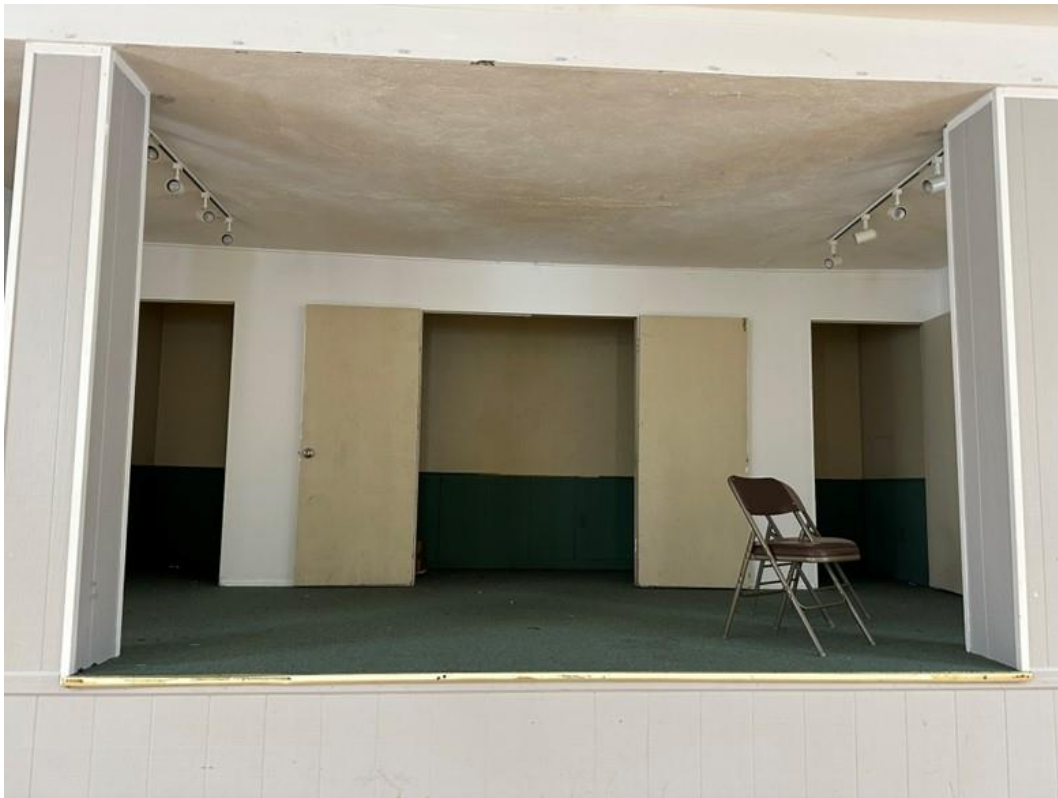
Photo 4: Deflection in Stage Ceiling
