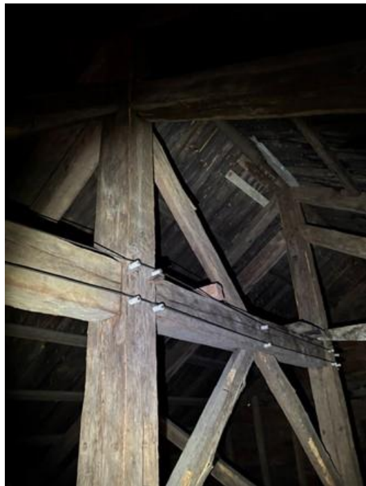
Photo 16: Missing brace in Main Truss
