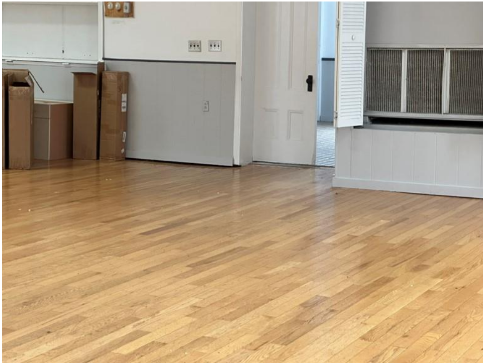
Photo 6: Deflection in Main Room Floor
