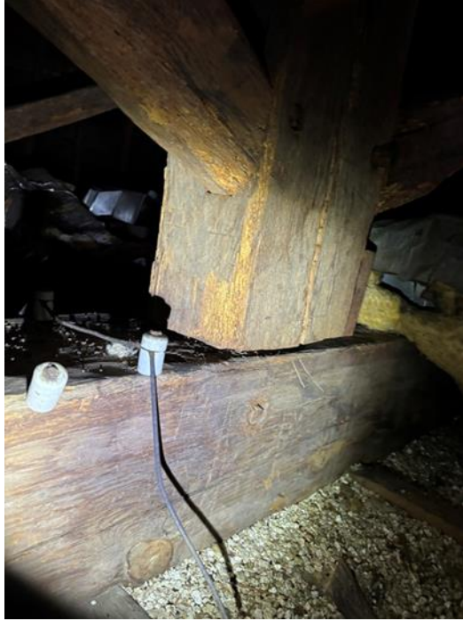
Photo 17: Powderpost beetle damage to trusswork
