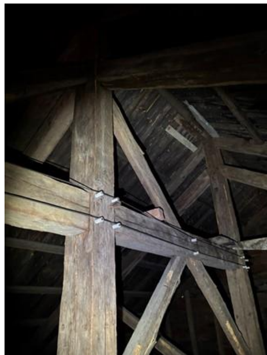
Photo 16: Missing brace in Main Truss
