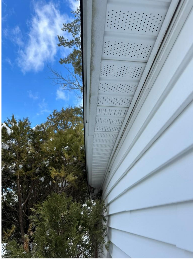
Photo 1: Outward bow in gutter of Side Room
