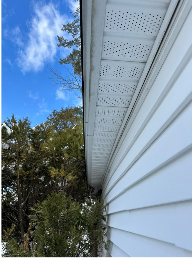
Photo 1: Outward bow in gutter of Side Room
