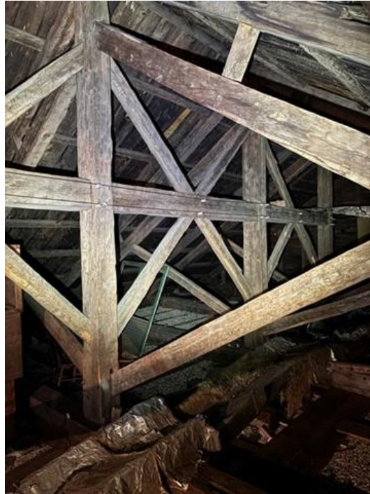
Photo 15: Missing brace in Main Truss
