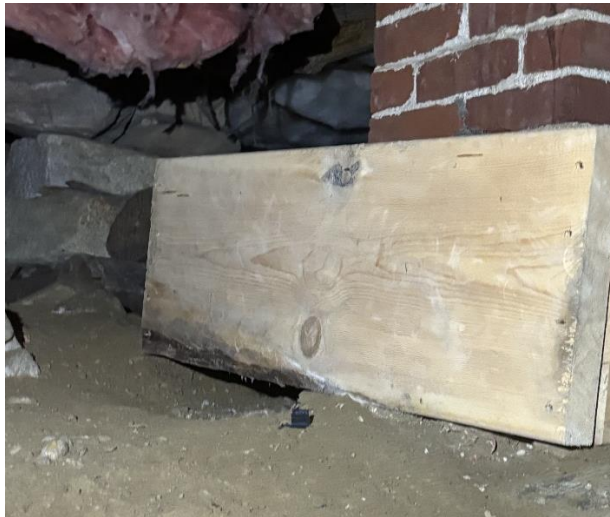
Photo 9: Burrow below pier
