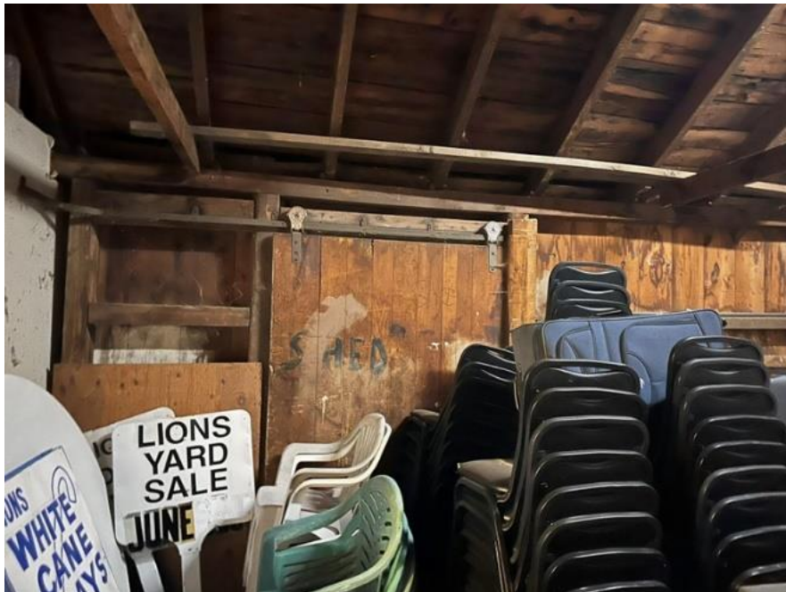
Photo 2: Deflection in Wall Plate of Side Room
