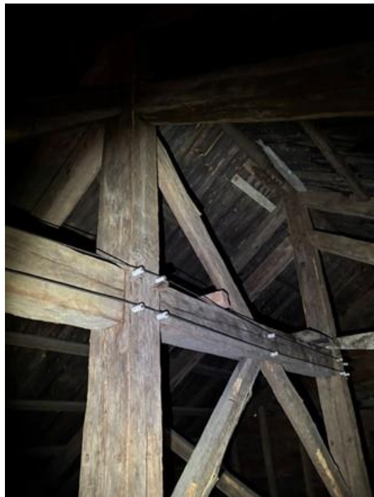
Photo 16: Missing brace in Main Truss
