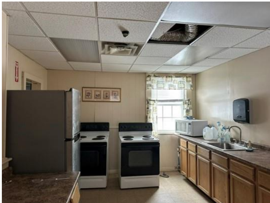
Photo 12: Deflection in Kitchen Ceiling
