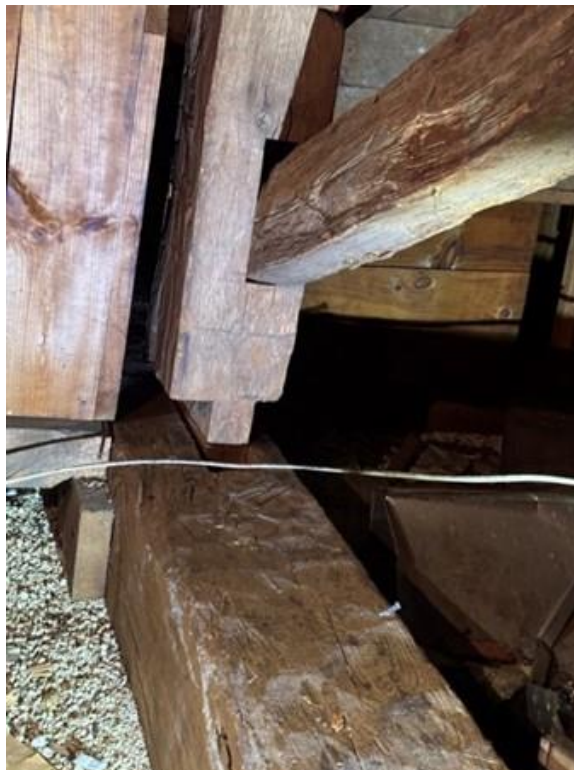
Photo 14: Deflection in Main Truss bottom chord
