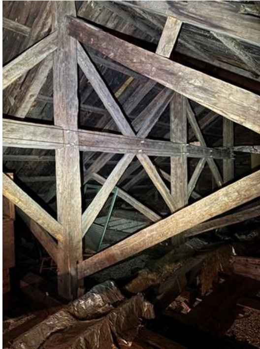
Photo 15: Missing brace in Main Truss
