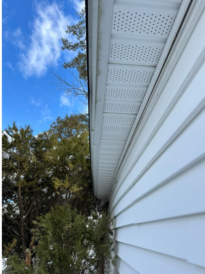
Photo 1: Outward bow in gutter of Side Room
