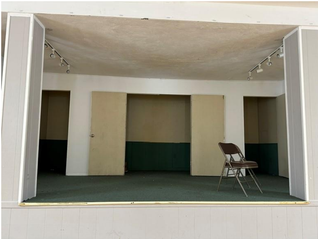
Photo 4: Deflection in Stage Ceiling
