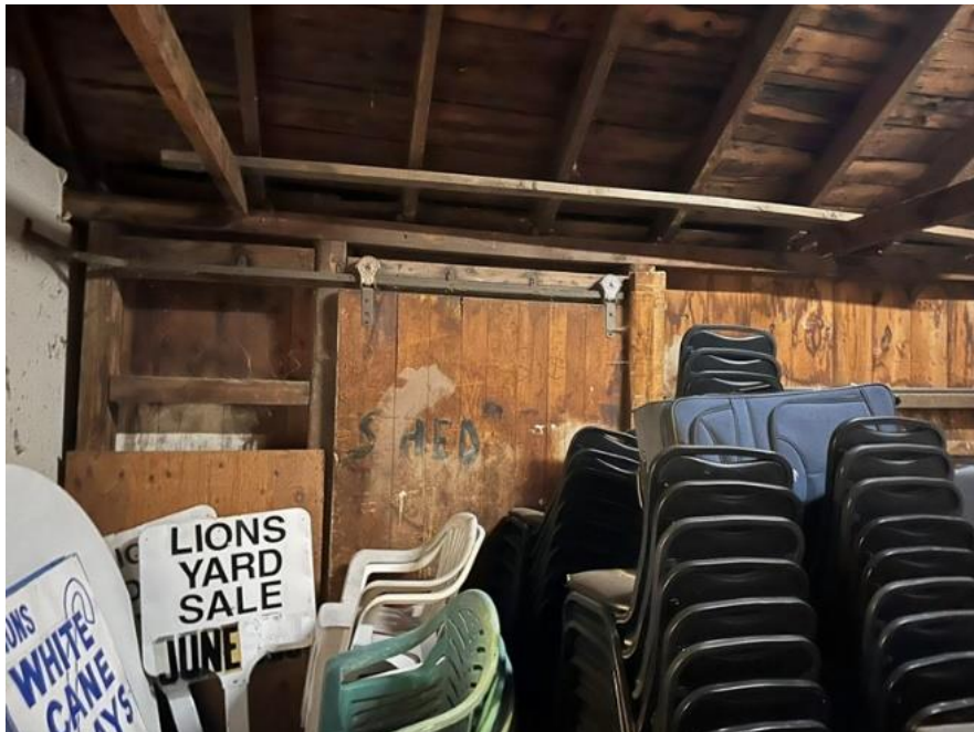
Photo 2: Deflection in Wall Plate of Side Room
