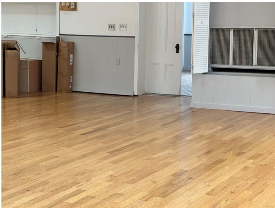
Photo 6: Deflection in Main Room Floor
