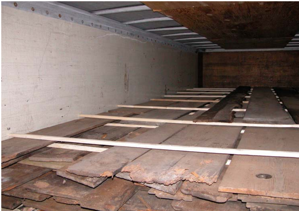
Subflooring and finish flooring boards are retained for reuse. Some repairs and in kind replacement will be necessary.
