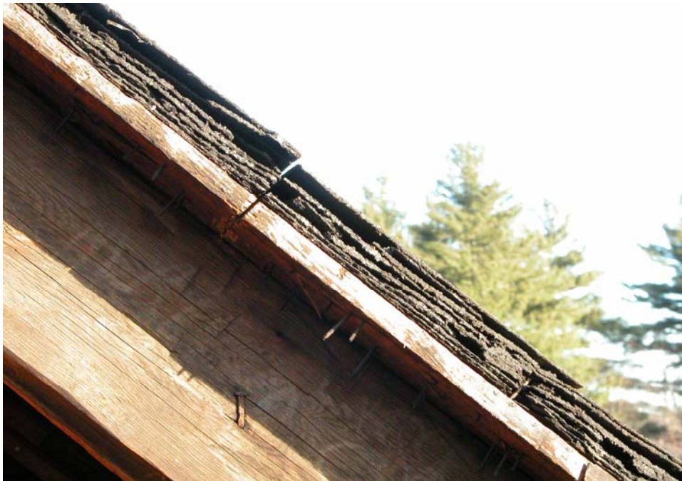
None of the roof sheathing was viable for reuse.
