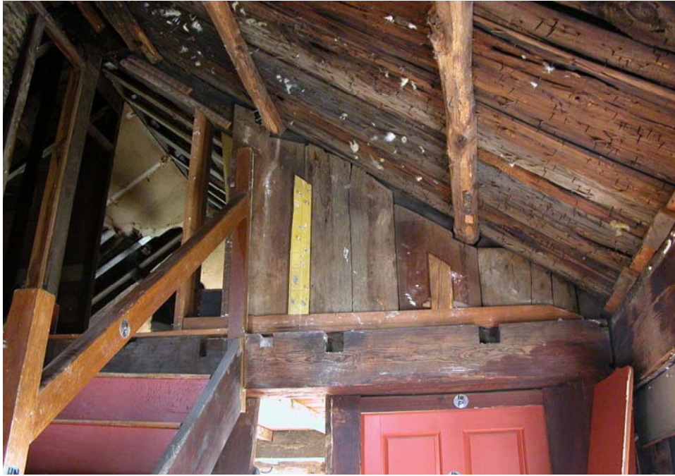
Roof boards in the Saltbox Ell and Main House had so many layers of shingles over them that they were cut out and discarded.
